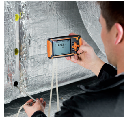
Pitot tube measurement in a duct
